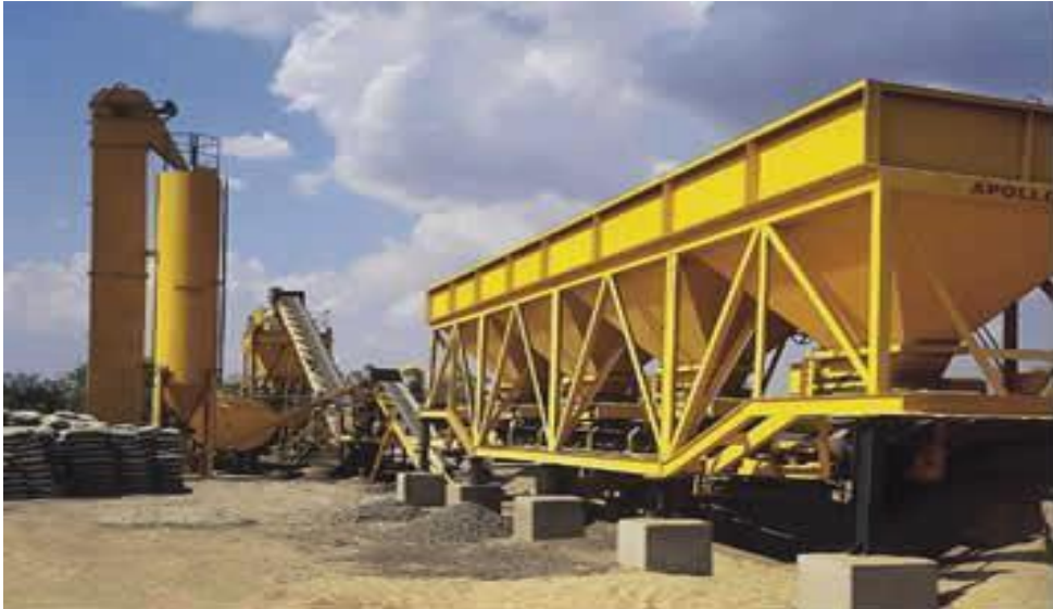
Fig-A5: Computer Controlled Bins for Mixing
