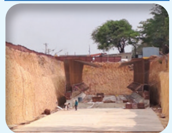
Channasandra box raft completed 45m out of 358m. Side wall (First lift) 90m complete out of 716m.
